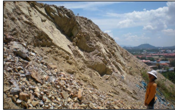
Figure 3: The slope rock mass forming a high density of plane discontinuities due to tectonic action. The rock mass is prone to disintegrate into varies size to the average size of 20cm resulting slope prone to failure.
