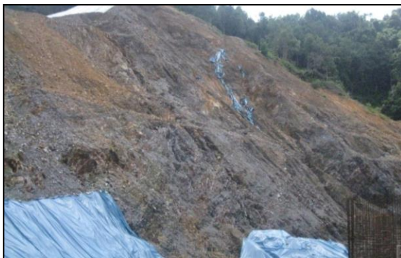
Figure 4: Gully erosion is observed because of surface water run-off. This failure becomes worse because no temporary erosion control measure was installed during construction stage.
